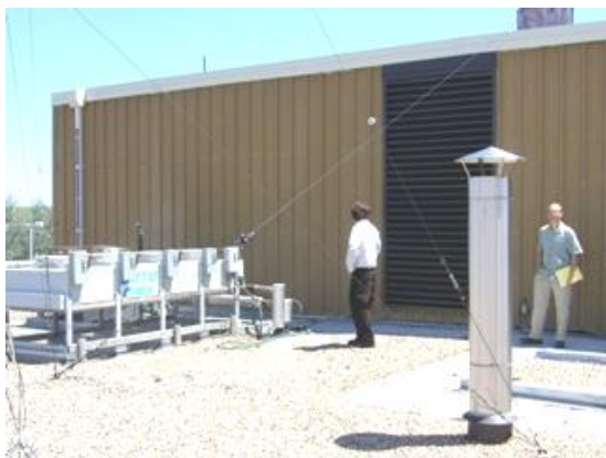
Figure 8. – EP 240 exhaust stack.
